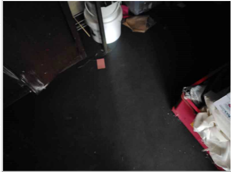
Photo No. 21 - Bitumen adhesive to floor below modern floor screed below modern vinyl floor sheeting
