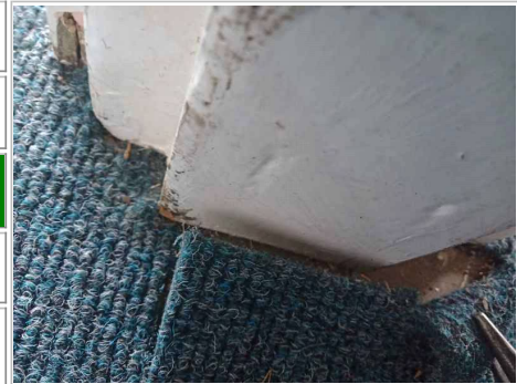
Photo No. 86 - Vinyl sheeting (grey) to window sills to south side of room (possibly blow new PVC window sill)
